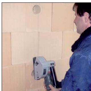
Use the wall chaser to cut slots in the JUWO POROTON Blocks.
