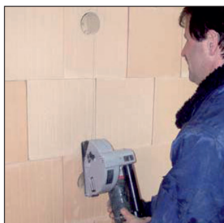
Use the wall chaser to cut slots in the JUWO POROTON Blocks.
