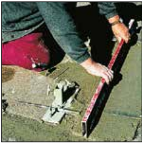
As with normal plane brick walls, the first layer is precisely placed in cement mortar M10.
