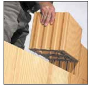
After the first layer of mortar has been placed, it is not filled yet, but the wall is created over its entire height with thin-bed mortar.
