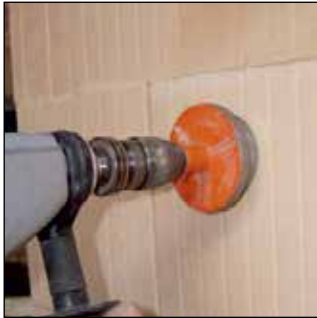
Mark the electrical socket and core drill with a conventional drill and diamond dry drill bit.
