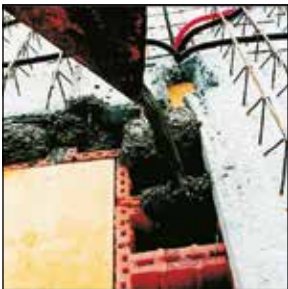
The plan filling brick is filled with concrete C12/15 (grain size 0-16, with BV). Then the ceiling can be concreted.
