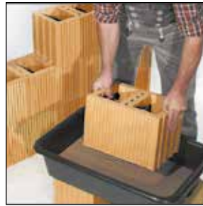
The thin-bed mortar mixed in the bucket is poured into the mortar pan. Here, brick by brick is briefly immersed, the mortar immediately adheres firmly to the underside of the brick.
