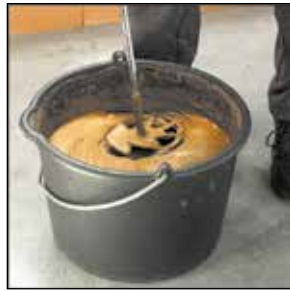
The thin-bed mortar is mixed with water and the whisk and then poured into a mortar trough for processing.
