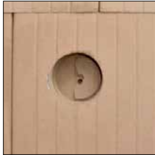
Remove any brick residue and drilling dust - and you have a perfect hole for an electrical socket.
