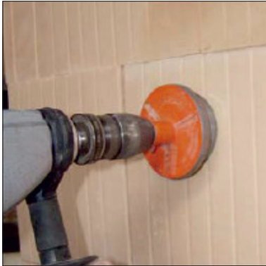
Mark around the socket outlet and drill a round hole using a commercially available drill and dry diamond core drill bit
